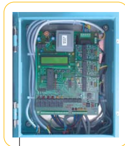
Remote monitoring interface
